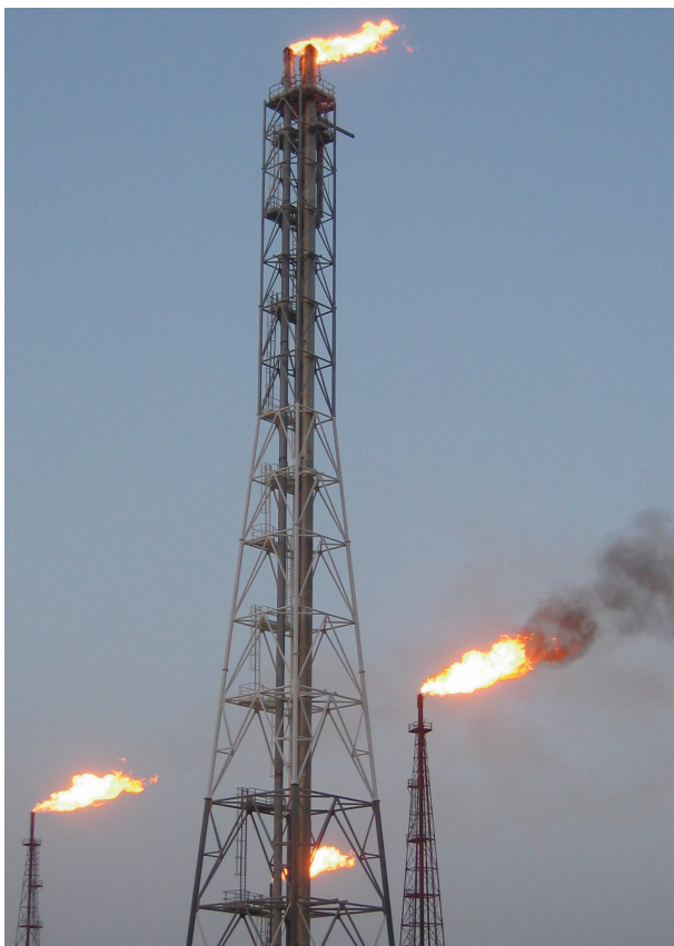
Figure 6. Flares in operation, with the three newest flares shown in the foreground.
